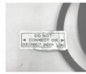
Warning Label attached on Cable
